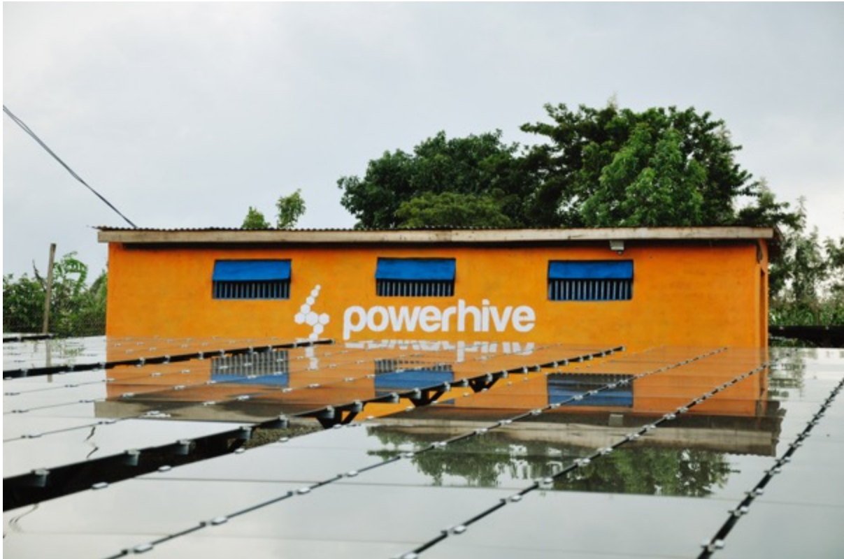
A functioning Powerhive microgrid, including solar panels and a central facility that houses batteries and inverters, at the village of Mokomoni in Western Kenya.
